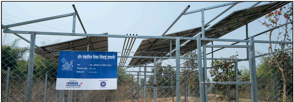
Solar Lift Irrigation
